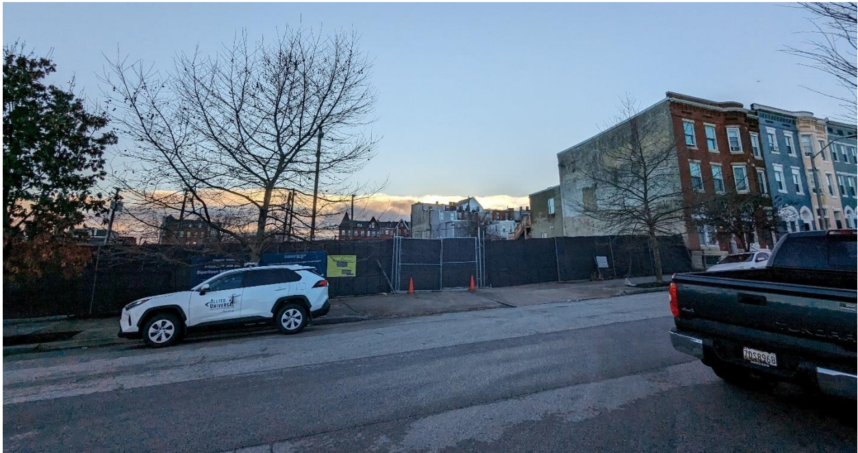
Fig. 27: 900 E. North Avenue and 2000 Linden Avenue are surrounded by construction fencing as buildings are demolished. View from across Linden Avenue.
